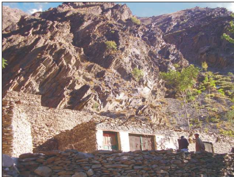
Fig 2.4: Vulnerable house located near steep cliff in Chitral
