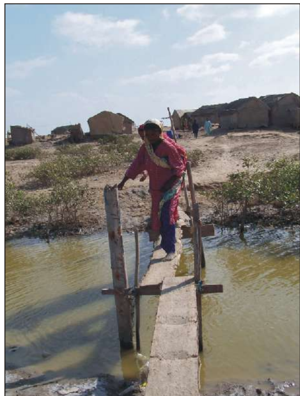
Fig. 2.11: An old women is crossing a broken bridge
